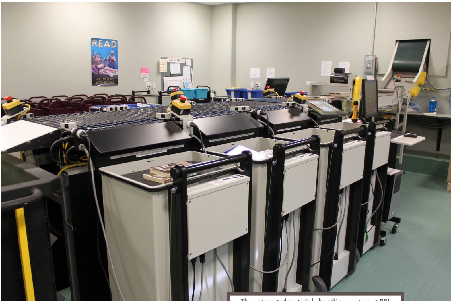
The automated materials handling system at PPL
